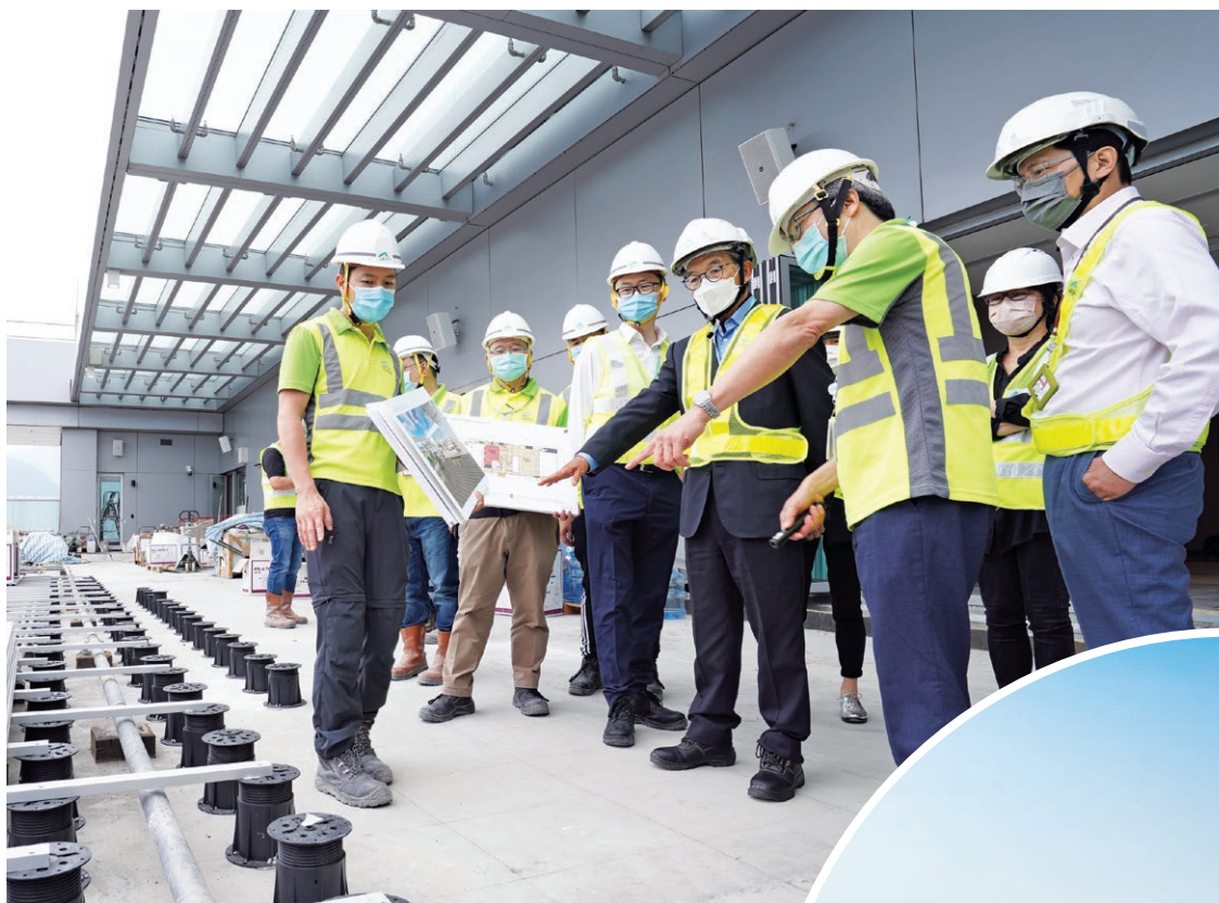
AA Chairman Jack So (fourth from right) is briefed on the progress of the HKIA Community Building. 機管局主席蘇澤光 (右四) 聽取機場員工綜合大樓的工程進度。
